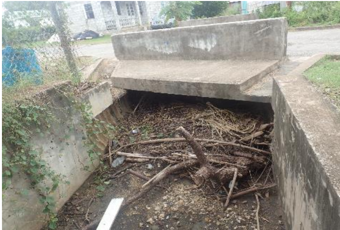
Photo 3: Debris blocking a road culvert, Barbados.
