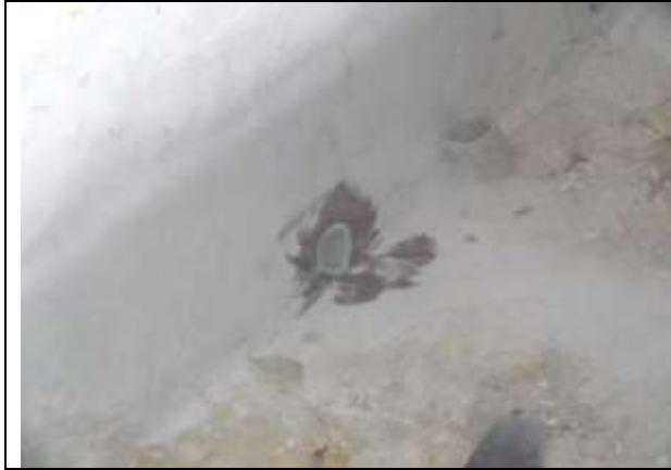
PVC 1 inch pipe drain; inside view.
